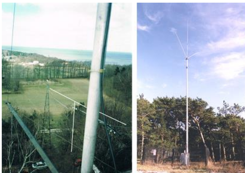
Fig. 4. The transmission antennas in the Rozewie (left side) and Dziwnów (right side) DGPS reference stations in 1995; in the photo of the Rozewie DGPS reference station the shape of its two wires (vertical and horizontal) are drawn with the white line; photos: C. Specht
